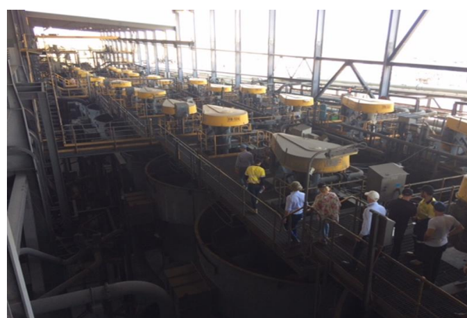
Source: Perennial Value - Flotation tanks at the Century processing facility
