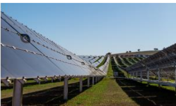
New Energy Solar’s Manildra Solar Plant Source: New Energy Solar
